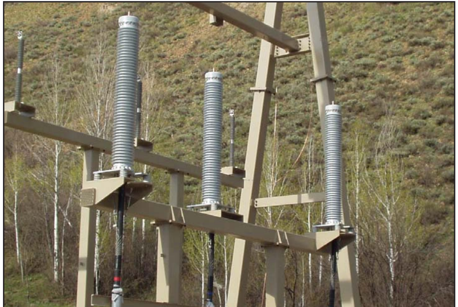
▲ G&W 245kV terminations with composite insulators
