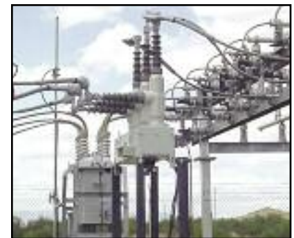
▲ Photo shows a custom mounted frame required for replacement of previously installed oil filled equipment.
