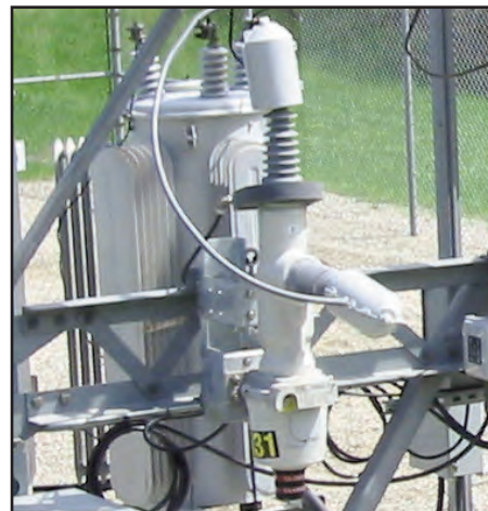
▲ Viper-ST reclosers with external CTs and wildlife protectors
