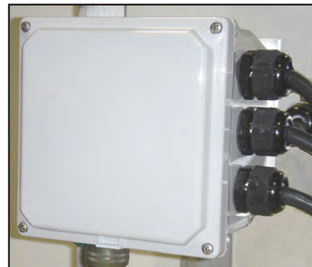
▲ Cabling from each recloser module is terminated inside a junction box permitting a single cable to go to the control. Cable entry can be using either strain relief or twist lock style connectors.
